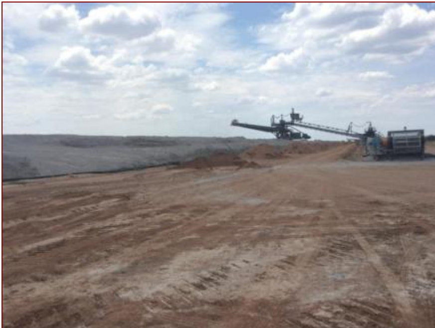
Figure 45- Machine that loads ash onto the facility from conveyor belt
